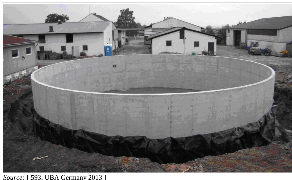
Figure 4.79: Underground slurry tank with liquid-tight geomembrane
